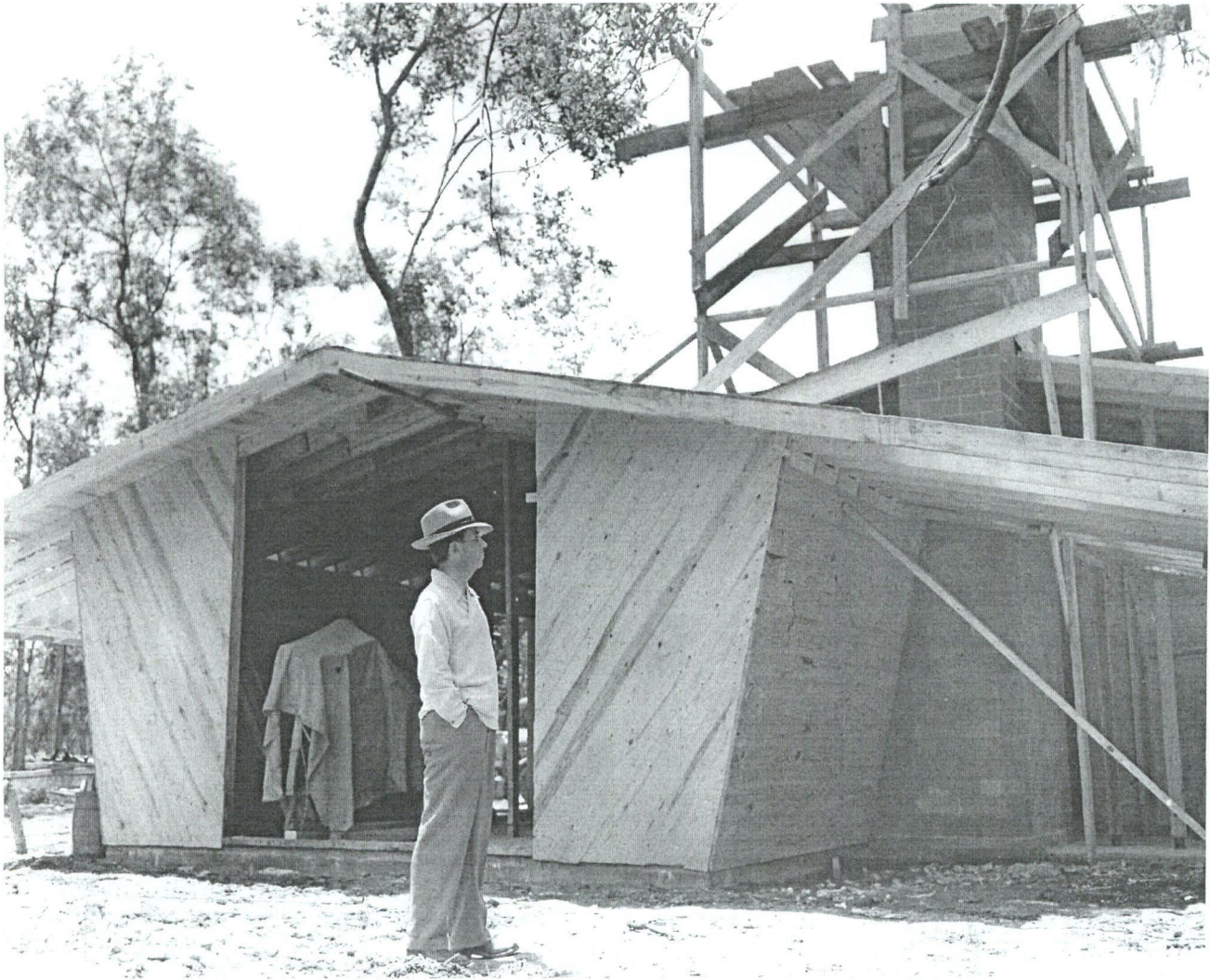
Photo 5. Alden B. Dow observing the construction of his office North Exterior, c. 1943
