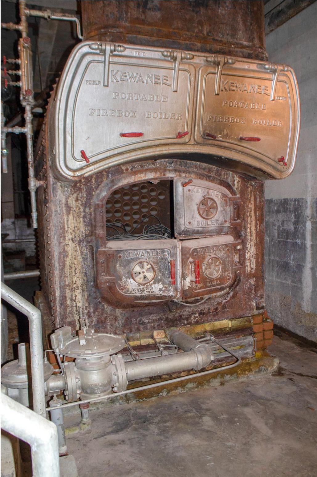
Photo 14: Boiler, view in basement. Camera facing east.
