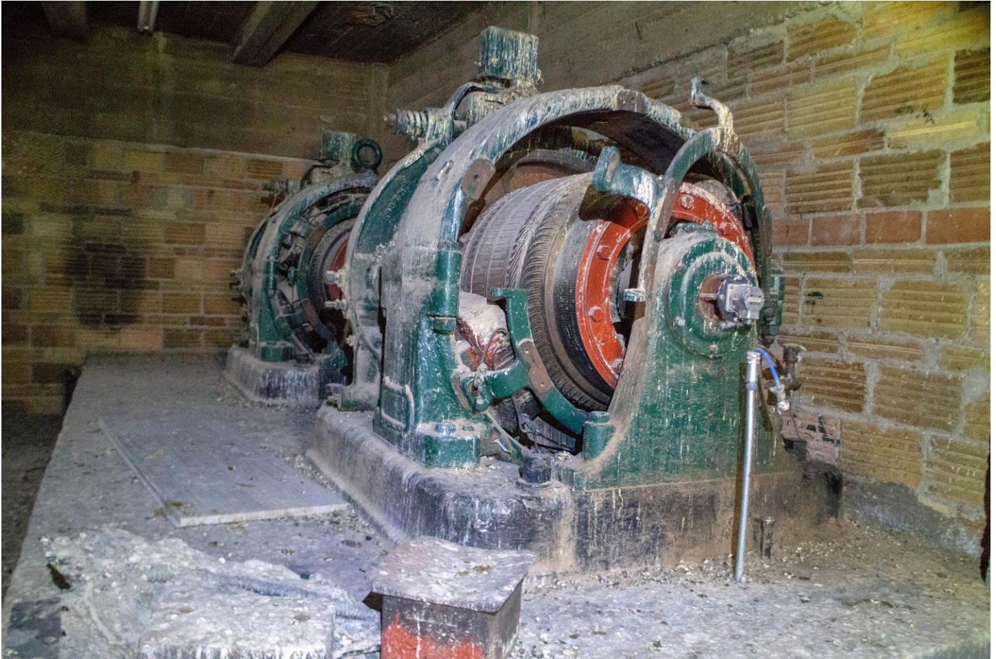
Photo 28: Elevator equipment in penthouse. Camera facing southeast.
