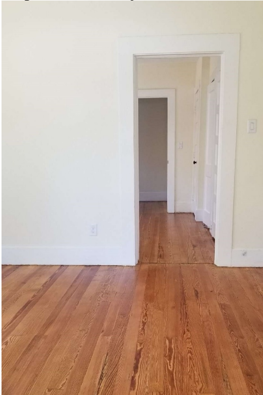
Photo 16: Interior living room showing entrance to rear rooms in 1219 Tulane. The interior plan with its characteristic bungalow circulation pattern is intact.
