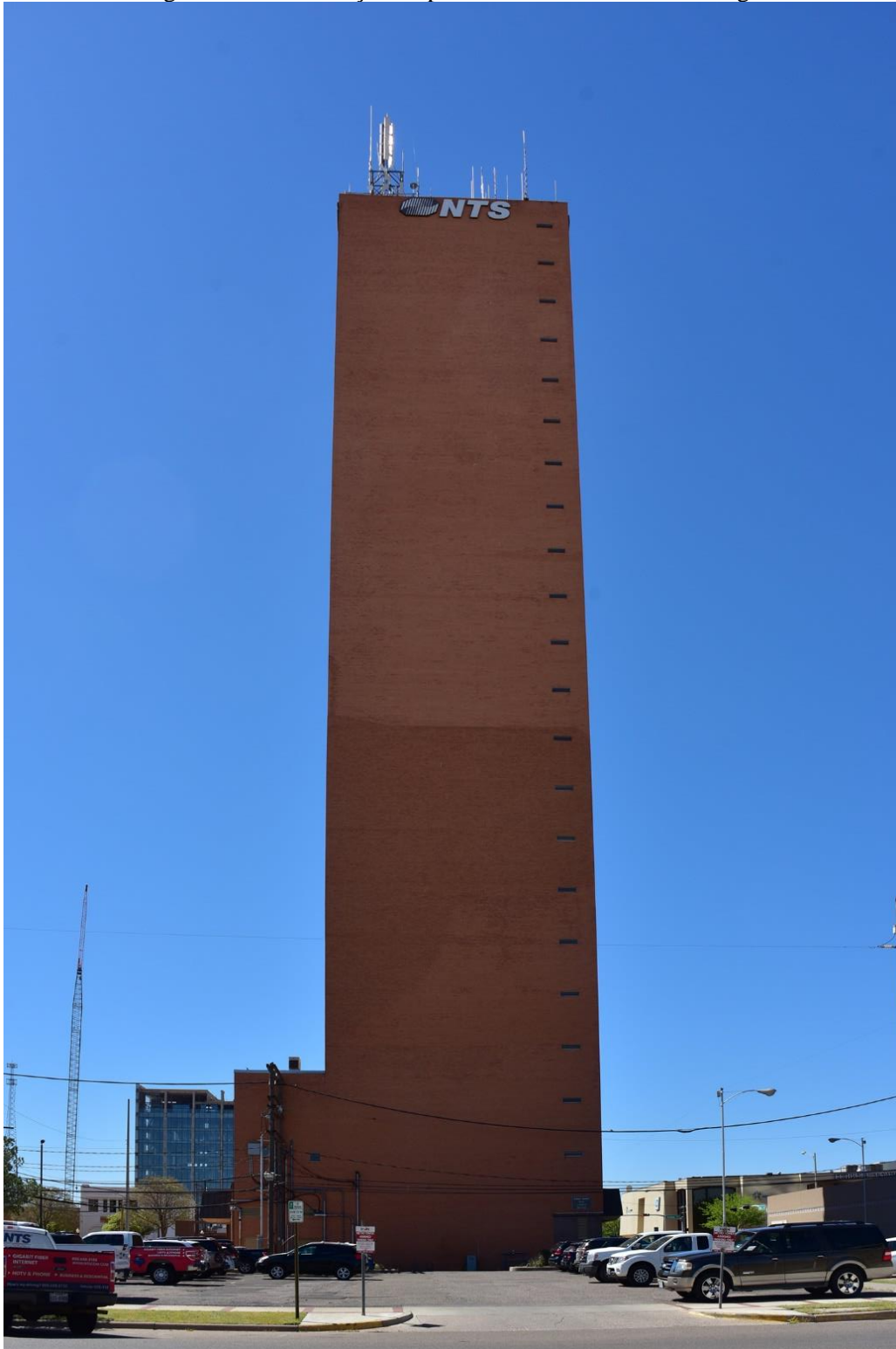
Photo 17. Facing brick on north façade repairs from 1970 tornado damage. Camera facing south
