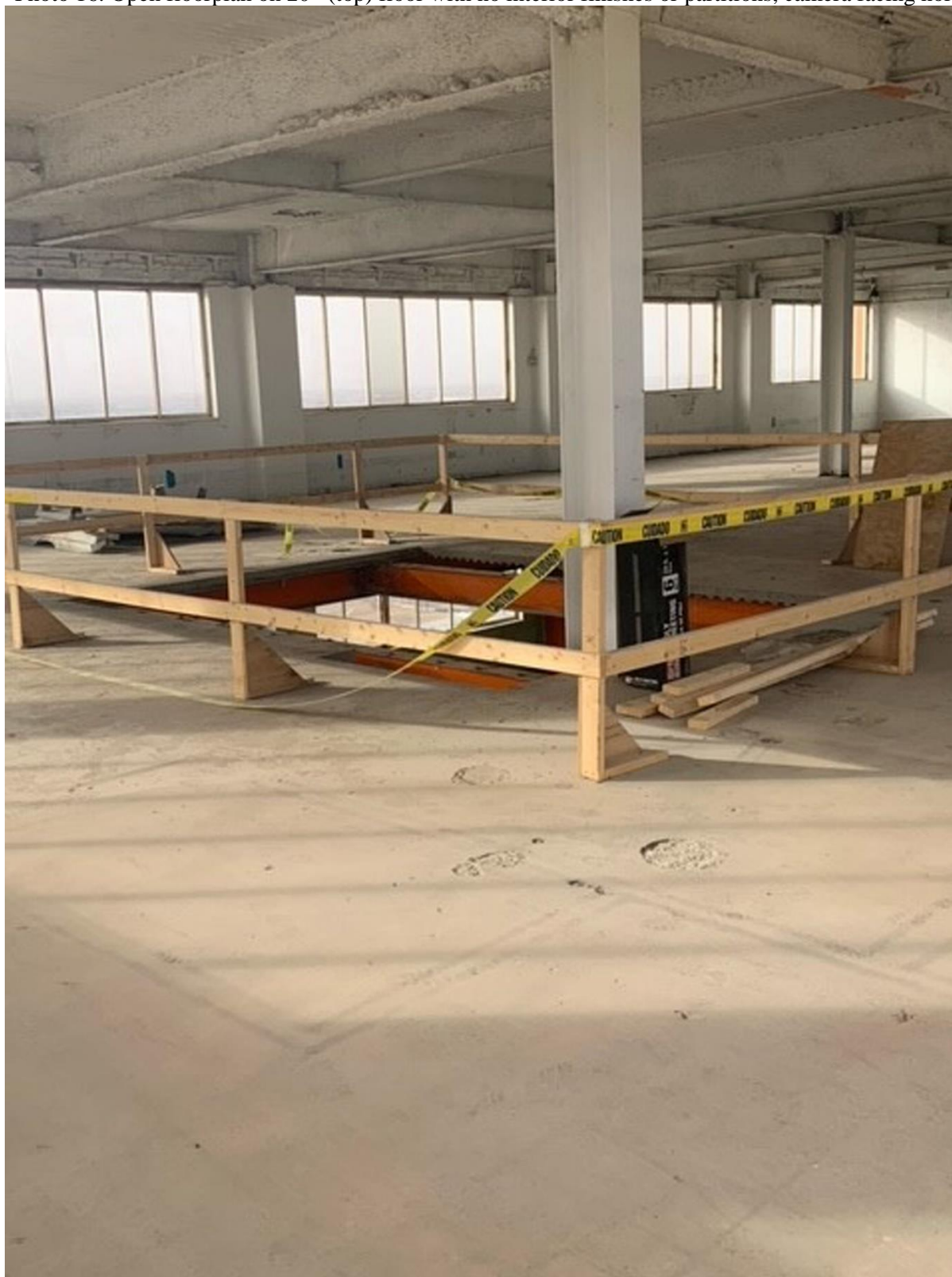
Photo 16. Open floorplan on 20 th (top) floor with no interior finishes or partitions, camera facing northwest
