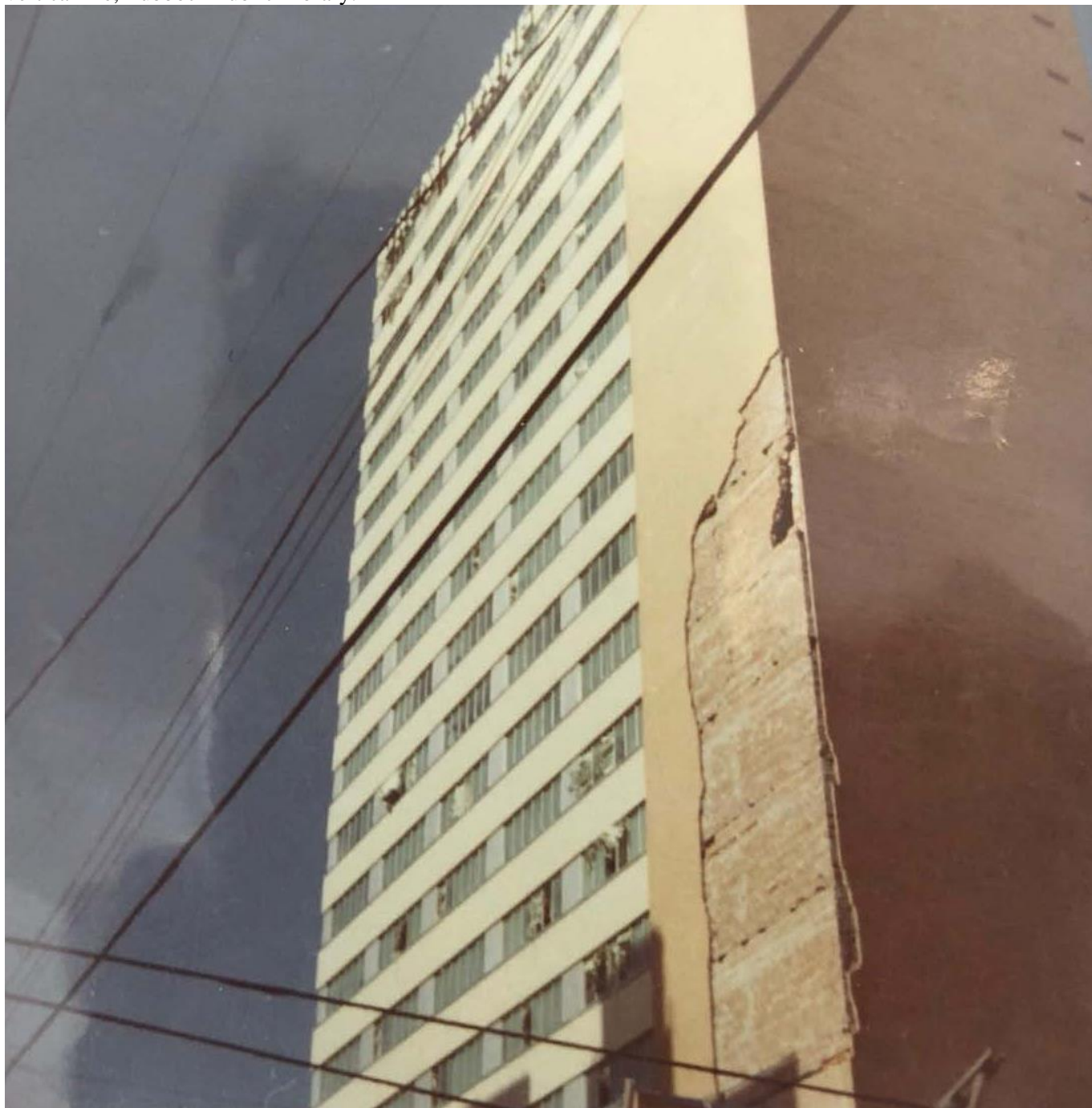
Figure 11. Historic Photograph of damage to northeast corner from 1970 tornado. Source: Lubbock Tornado vertical file, Lubbock Public Library.
