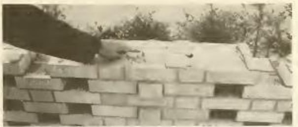
Photograph 29—Overturning of wall occurred at level at which vertical reinforcement was terminated. (Location 14)
