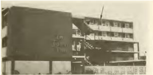
Photograph 27—South elevation of five-story motel with damage to glazing in upper floors. (Location 14)
