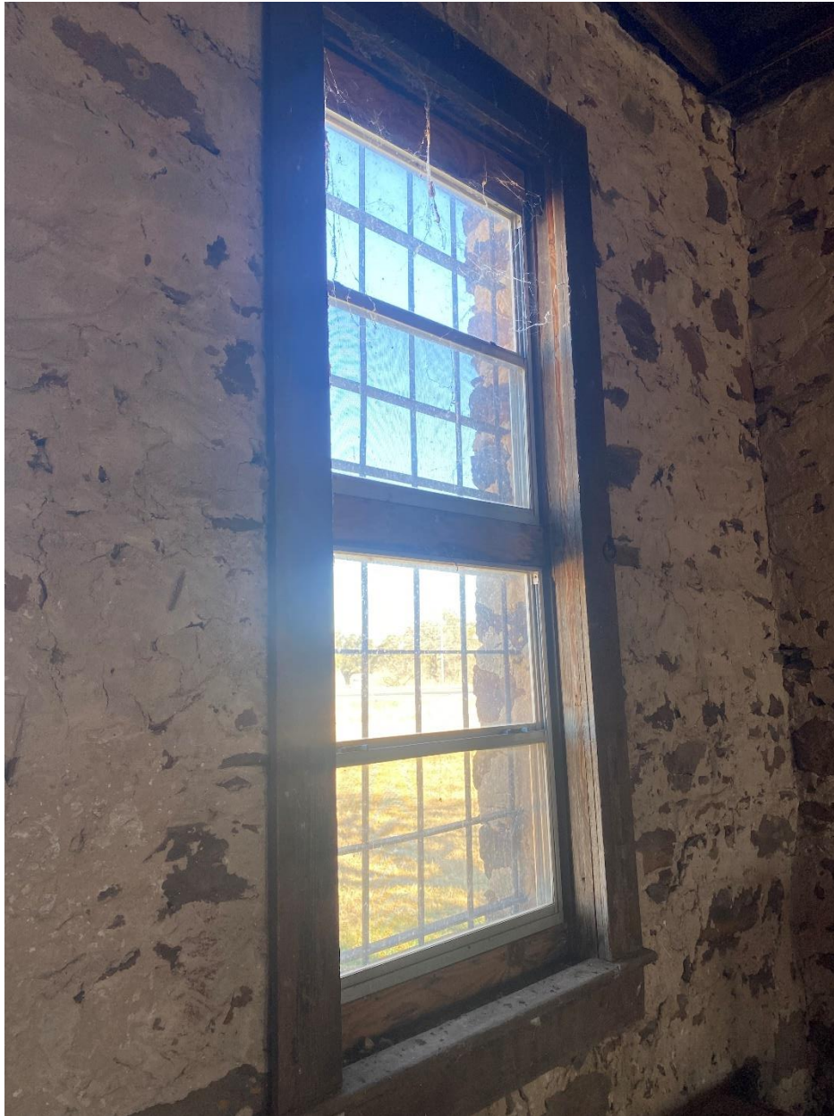
Photo 10: Replacement window in original openings, Heermann Store.
