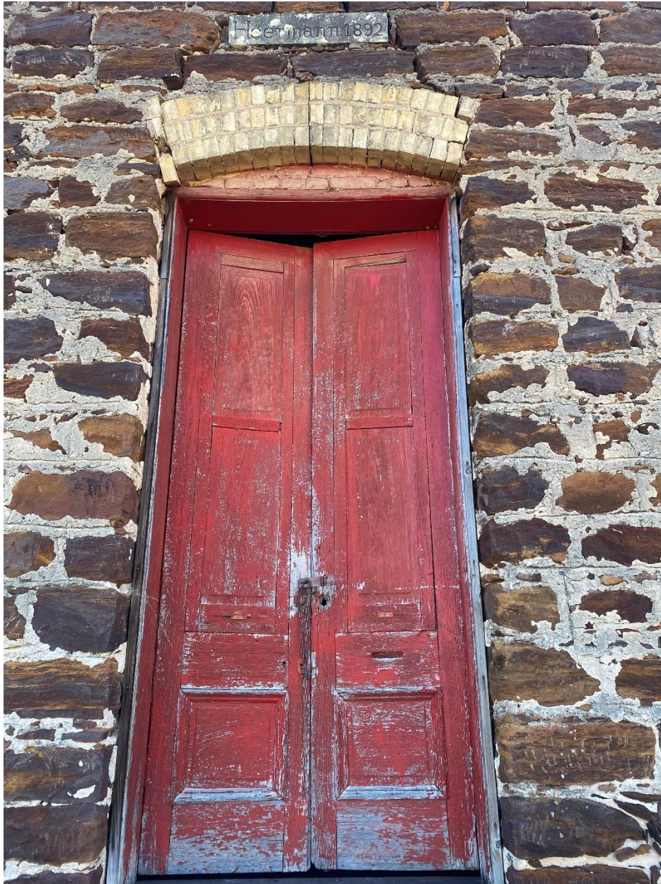
Photo 2: Primary (west) elevation of Heermann Store showing main entrance, camera facing southeast.
