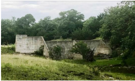
Concrete Dam (12a) – This board-form concrete dam is about 25 feet tall and approximately 55 feet long along its crest. The dam has three fin-like buttresses on the downstream side. It is not currently in use.
