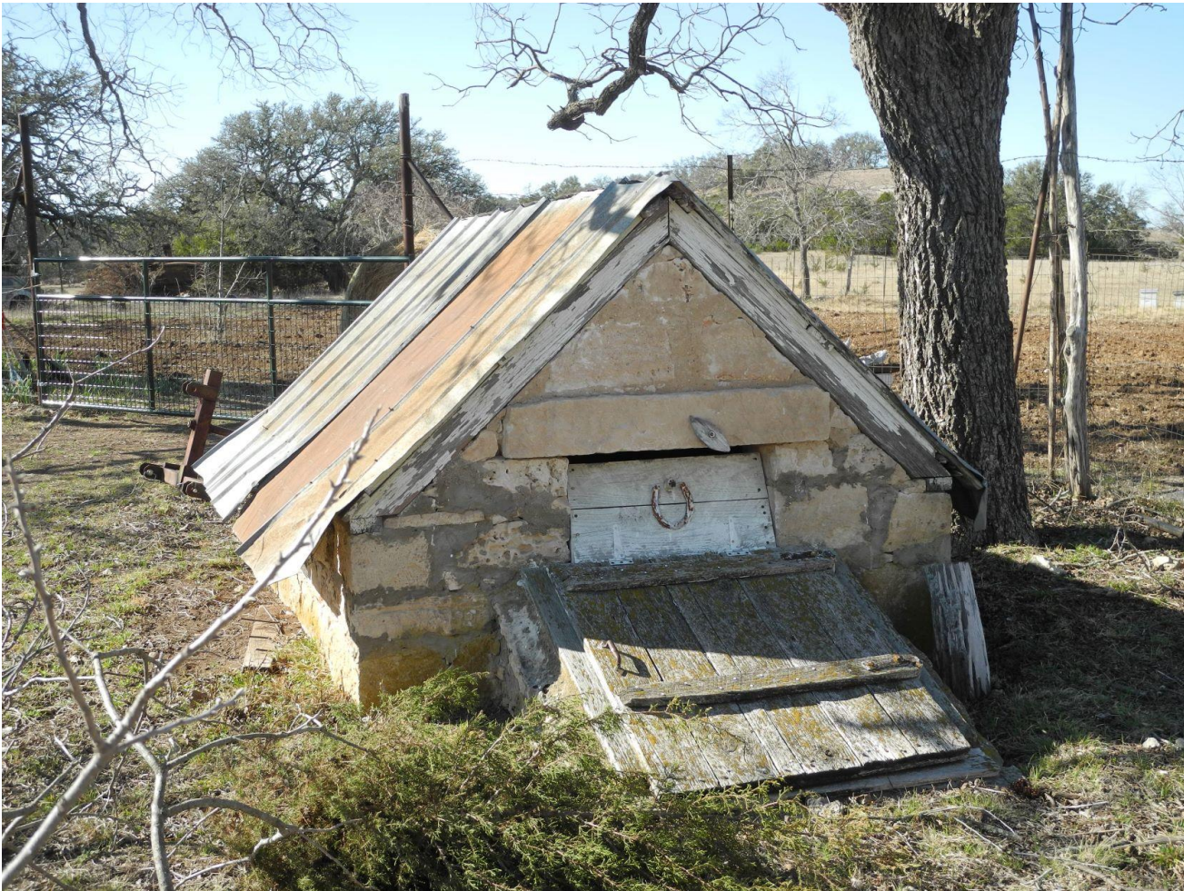
Photo 7: Contributing Building. Stone Storm/Root Cellar (Resource 2j), built 1902, Feuge Farm. Photo by Terri Myers, March 10, 2022, camera facing northwest.
