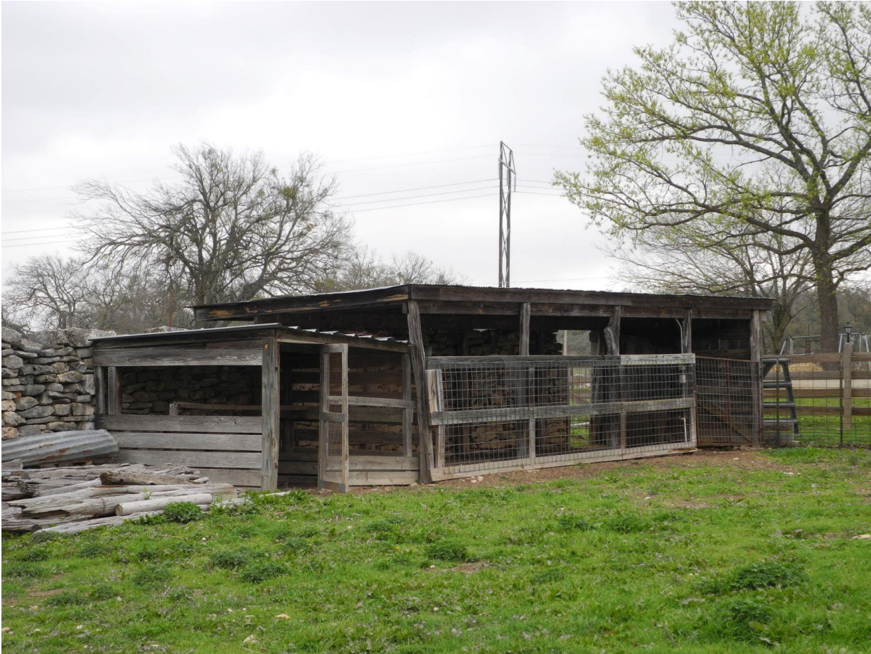
Photo 23: Contributing Building. Stone and Frame Livestock Shed (Resource 6f), c. 1860/1928, Amandus Stehling Farm. Photo by Terri Myers, March 25, 2021, camera facing southeast.
