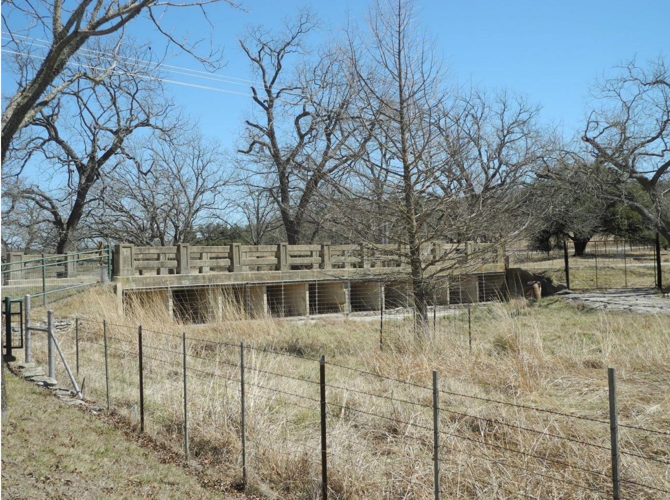
Photo 30: Contributing Structure. WPA Bridge on Old Mason Road (Resource 7a), c. 1935, Paul Stehling/Amandus Stehling Farm. Photo by Terri Myers, March 12, 2022, camera facing east/southeast.
