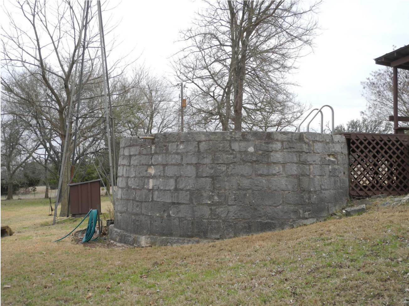
Photo 18: Contributing Structure. Stone Water Tank (Resource 3d), c. 1889, George Franz Stehling Farm. Photo by Terri Myers, March 11, 2022, camera facing northwest.
