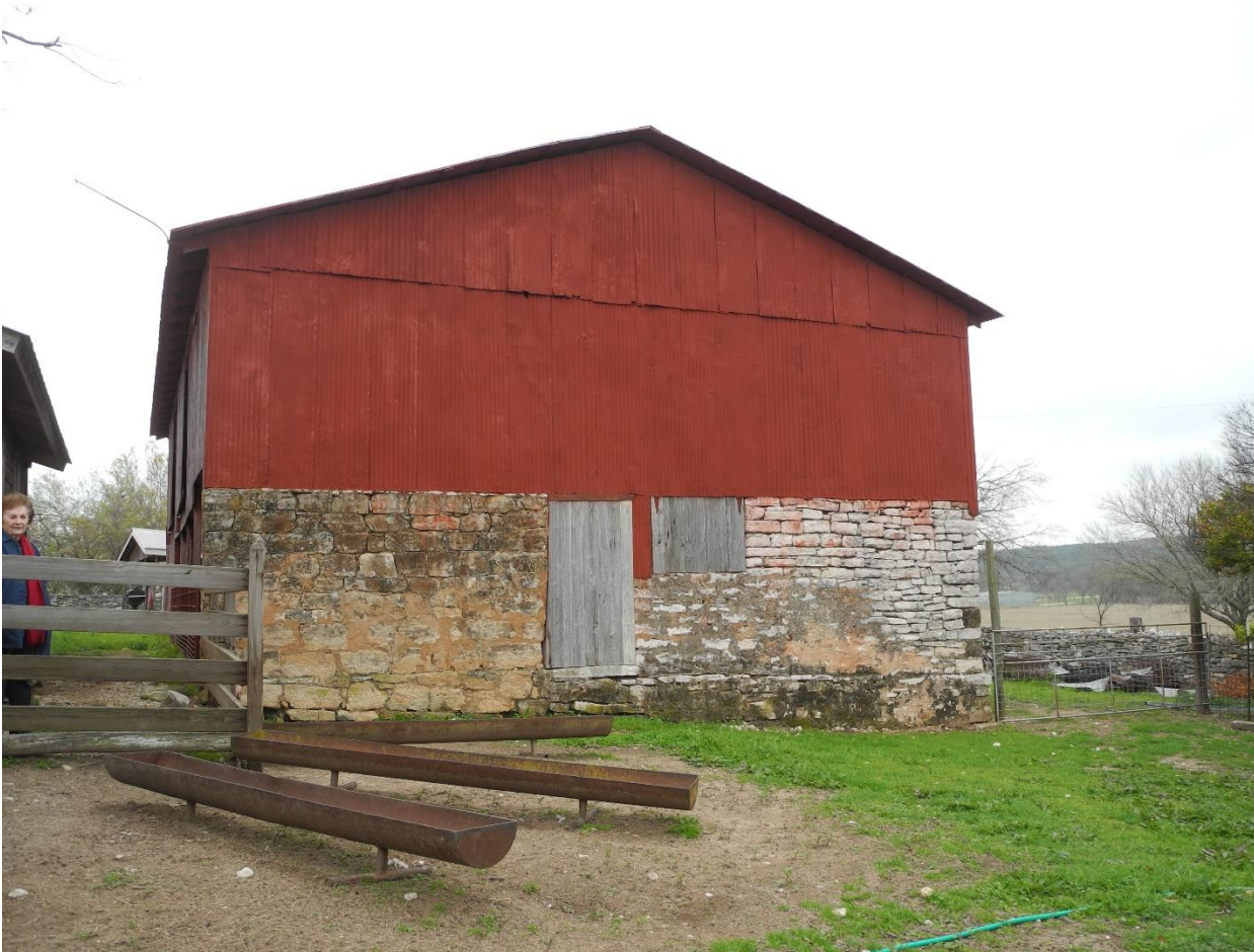
Photo 57: Materials and Methods. Original barn burned in the 1930s, but the stone foundation and some of the stone basement walls survived (left side). New walls built with remnant stone. Photo by Terri Myers, March 25, 2021, camera facing west.
