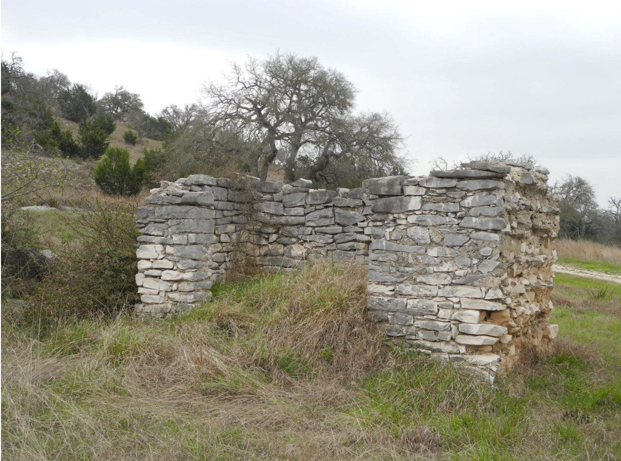
Photo 29: Contributing Site. Ruins of Thiele House (Resource 14e), c. 1852, on land later acquired by Amandus Stehling. Photo by Terri Myers, March 25, 2021, camera facing northeast.
