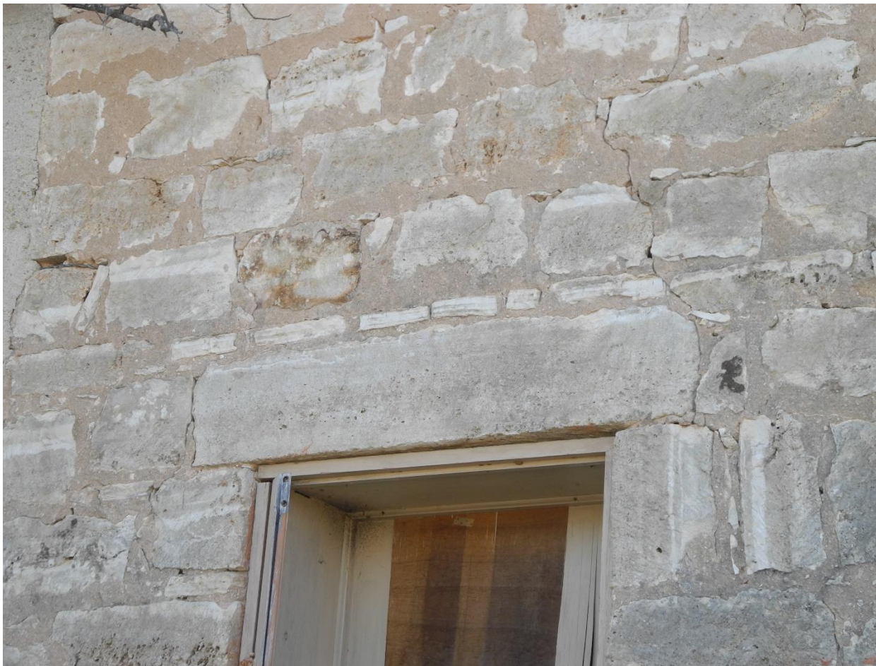
Photo 54: Materials and Methods. Christoph Feuge (Jr.) House, c. 1870, window detail. Cut stone lintels with row of small stones as chinking. Photo by Terri Myers, March 10, 2022.
