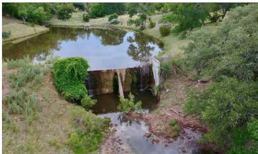
Concrete Dam & Pond (12d) – This board-form concrete dam is about 25 feet tall and approximately 85 feet long along its crest. The dam has earthen and concrete abutments at each end and one fin-like buttress on its downstream side. The pond created by the dam is 3/4 acres in size and has a wood fishing pier at its west bank.
