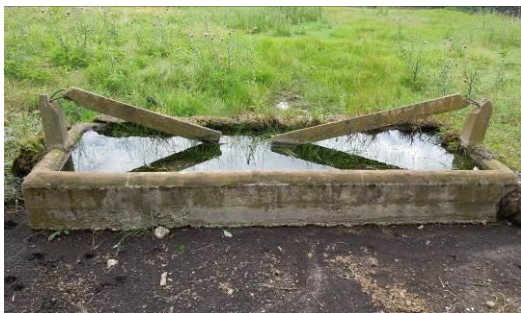
Spring-Fed Trough (12b) – This spring-fed trough is a rectangular concrete structure with side walls rising only a few inches above grade. The trough had a concrete rail above it, but the rail broke near its center point and collapsed into the basin.
