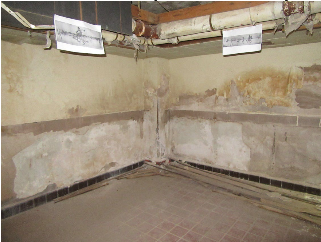
Photo 11: Basement, deteriorated H.D. Bugbee mural in the Old Tascosa dining room, looking southwest.
