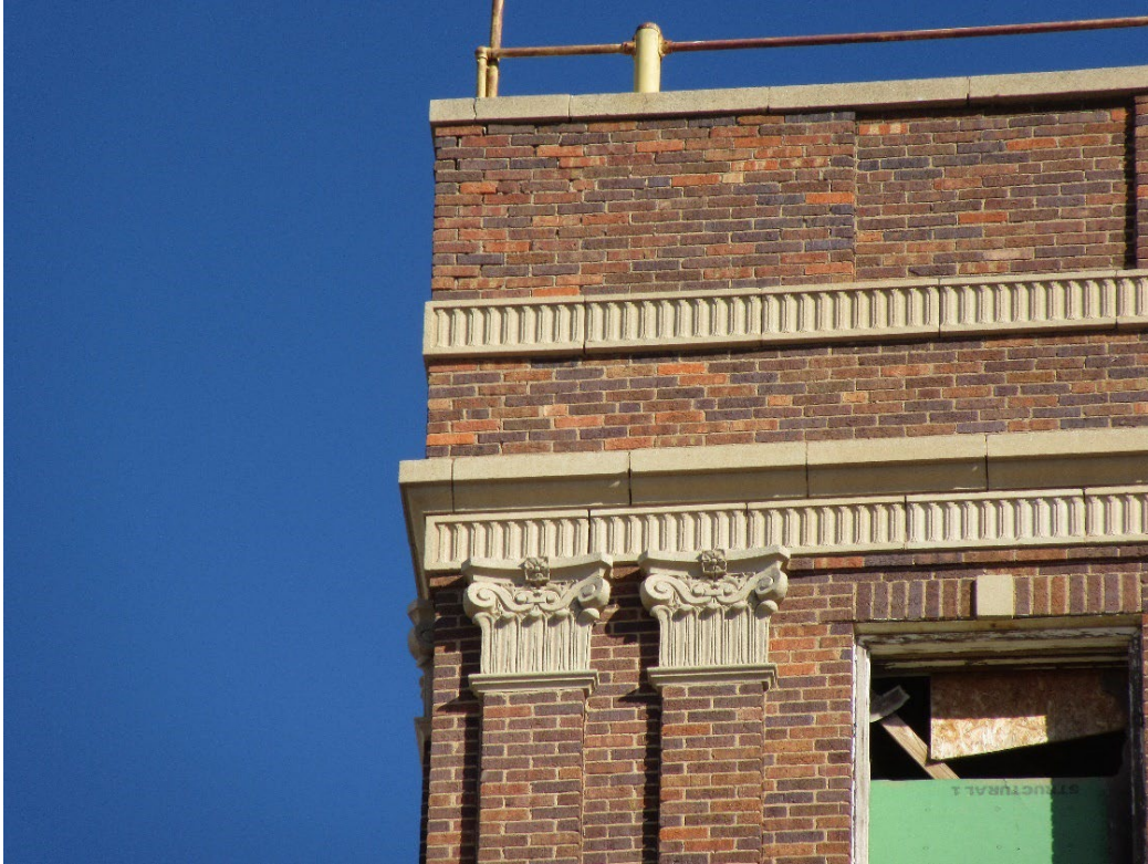
Photo 4: South elevation, decorative cast stone details at the top of the building, looking north.
