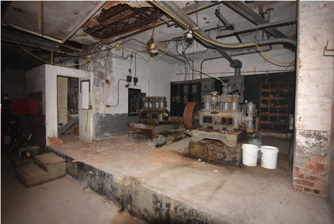
Photo 21. Interior, Carrier-Brunswick compressors in mechanical room, view facing southwest.
