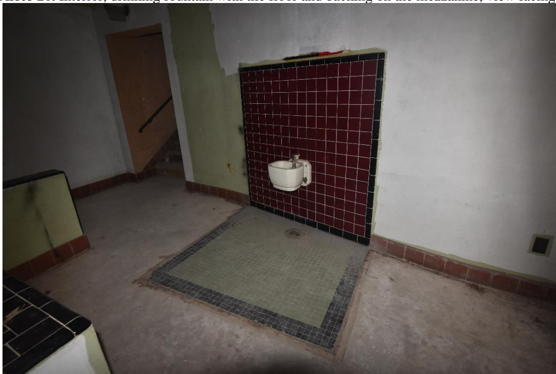
Photo 20. Interior, drinking fountain with tile floor and backing on the mezzanine, view facing northwest.
