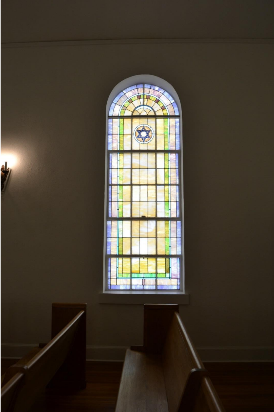
Photo 15. Detailed view of stained-glass window on east wall of sanctuary. Camera facing east.
