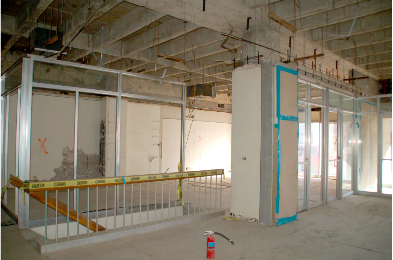
# 13 - Interior view, east corridor and staircase leading to basement, camera facing northeast
