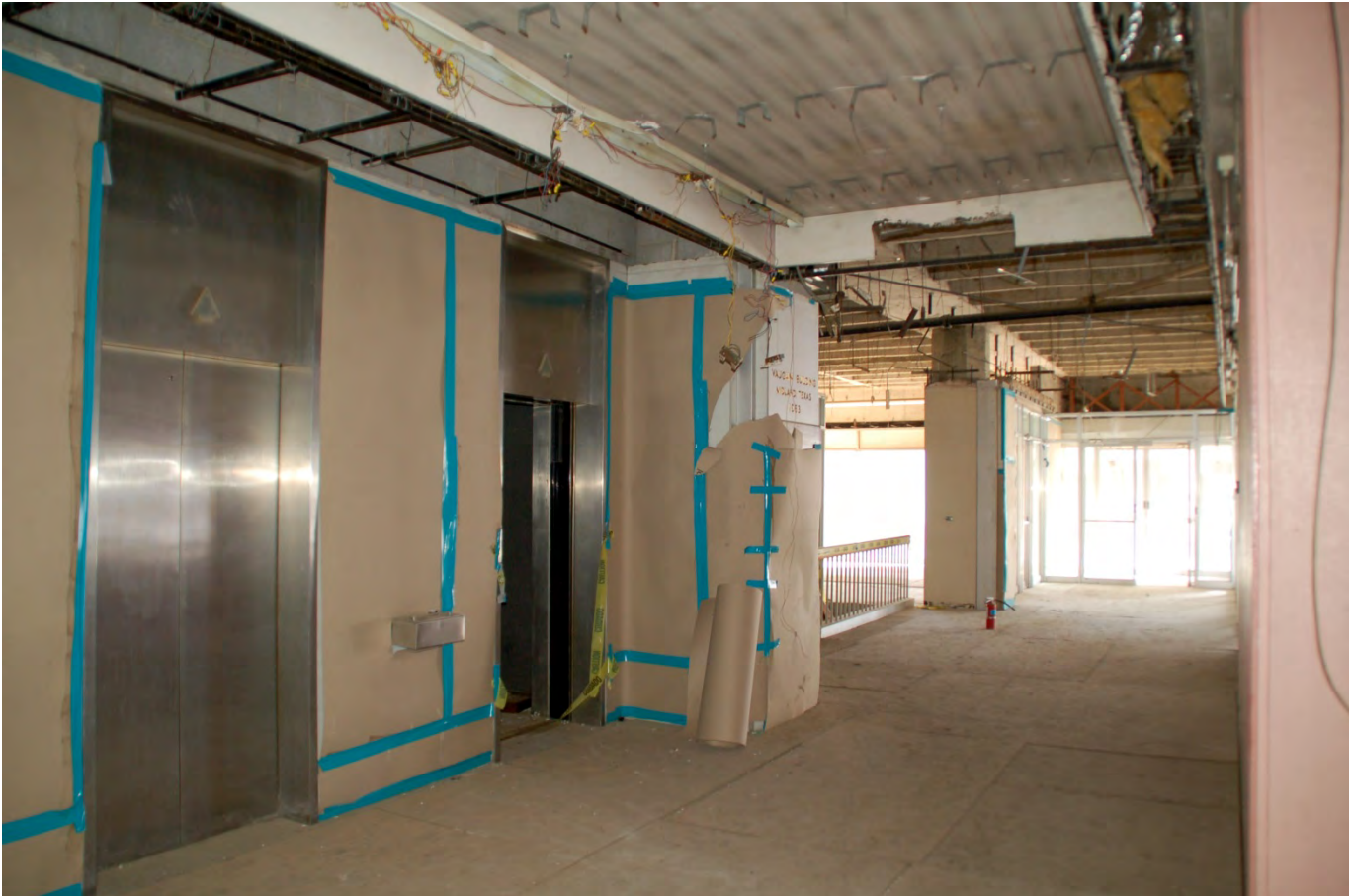
# 12 - Interior view, first-floor elevator lobby and east corridor leading to east building entrance, camera facing northeast
